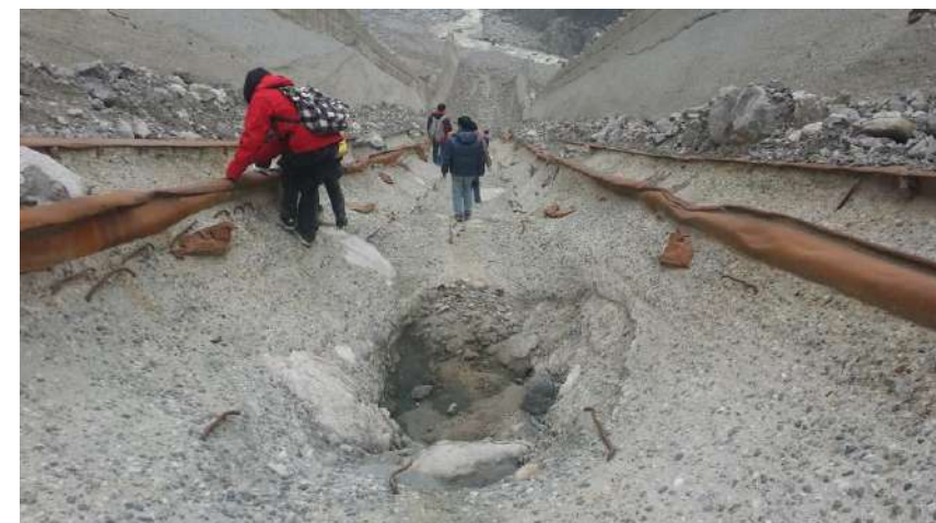
Eroded debris flow diversion channel (Xiaogangjian gully)
