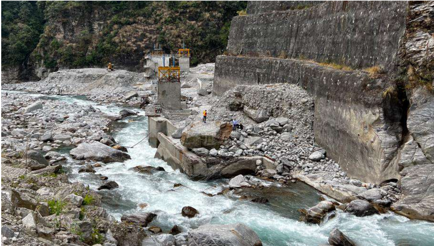
Melamchi water supply intake in November 2022
