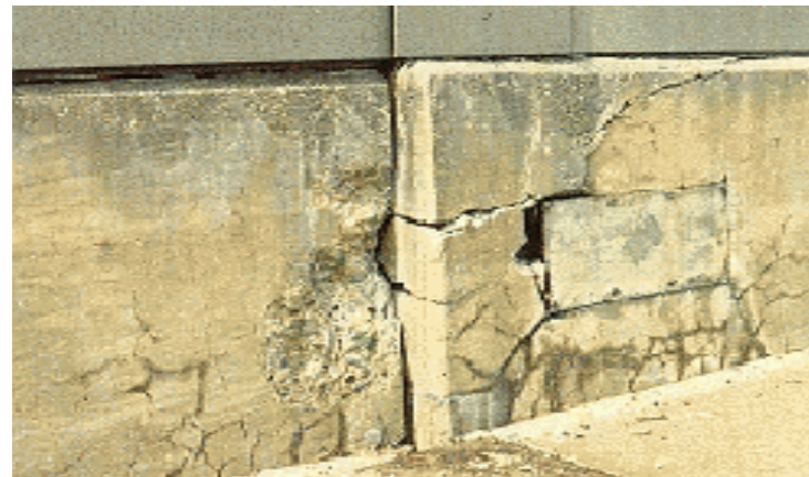
AASHTO Innovative Highway Technologies
