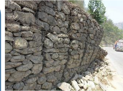
Gabion retaining wall tilted inconsistently by the earthquake
